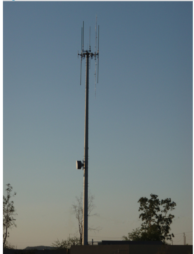
Figure 2.11. Antenna Tower and Antenna
